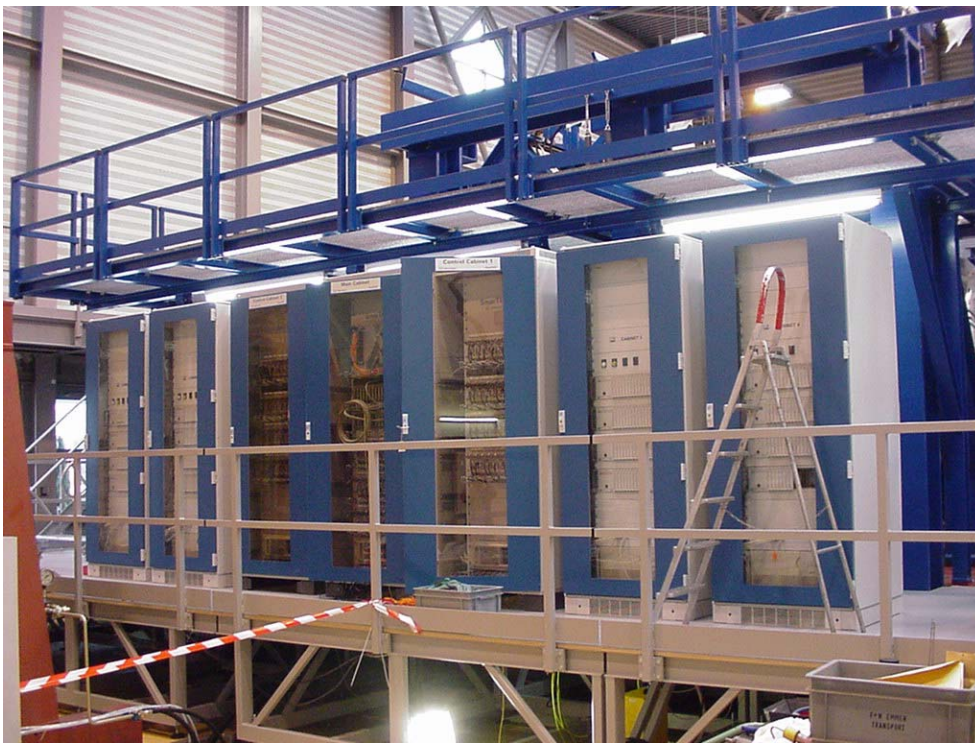
Figure 4.7_4: Racks for the control and monitoring system (middle three) and the data aquisition system (two left an rigt)
