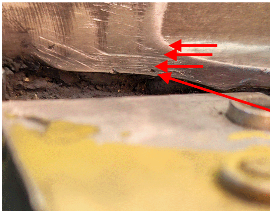
Figure 7: Crack From a Gouge in a Fracture Critical Part
