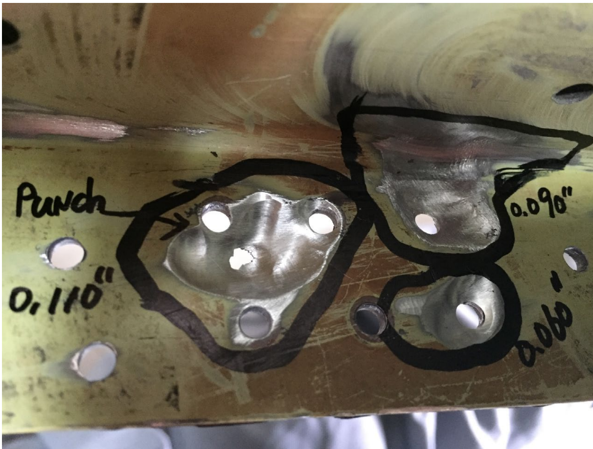
Figure 6: Corrosion Damage and Perforation
